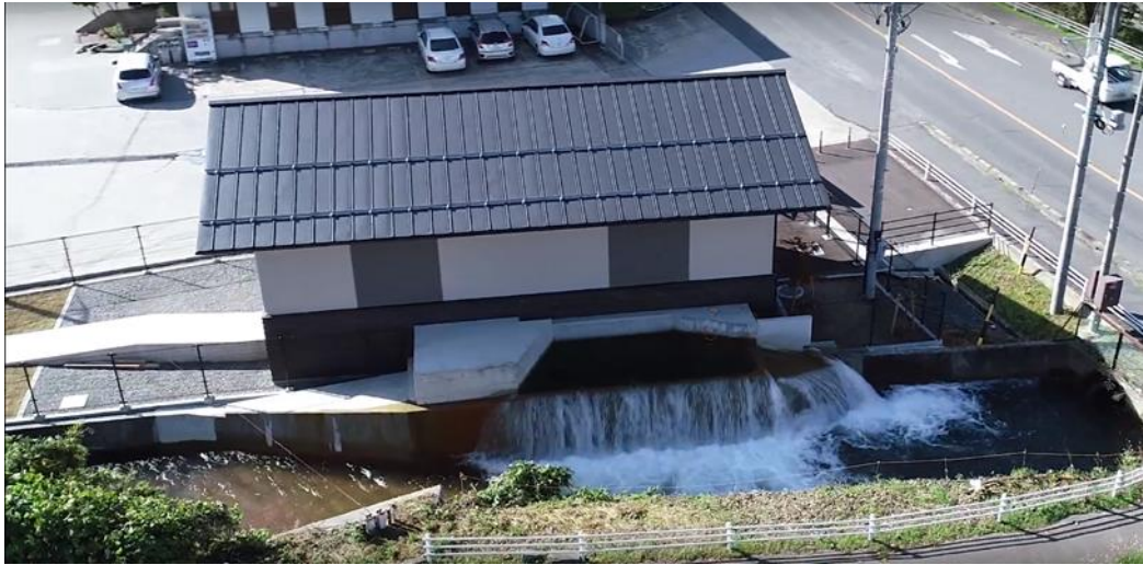
[The Obuse Matsukawa small-scale hydroelectric plant: external views of the turbine (upper) and building (lower)]
