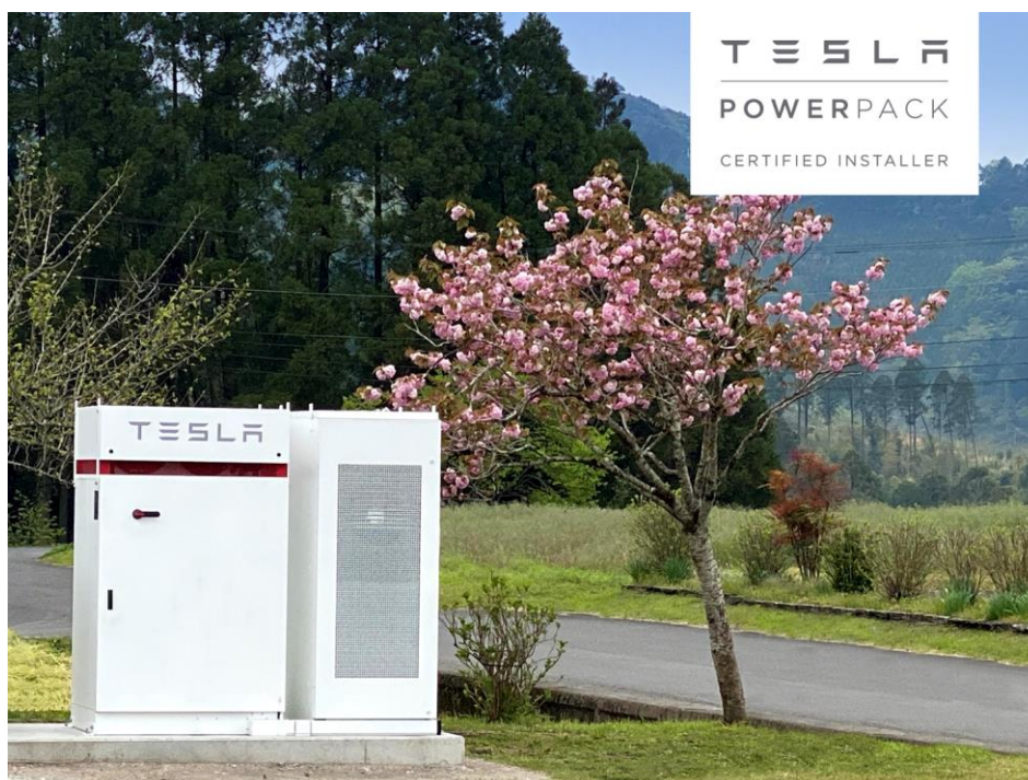
Installed Tesla Powerpack storage batteries (Shizen Energy is one of Powerpack Certified Installer for its industrial use storage batteries by Tesla.)
